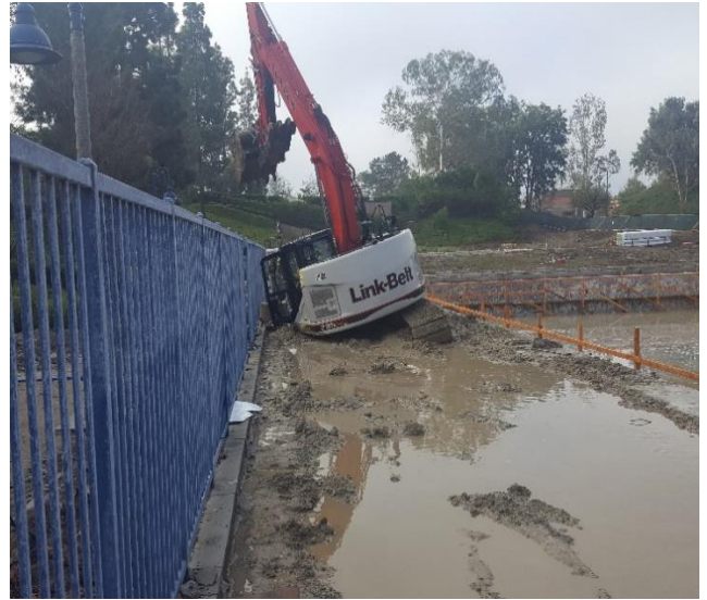
EXCAVATOR STUCK IN MUD AFTER STORM TRYING TO EXCAVATE AND KEEP PROJECT MOVING
