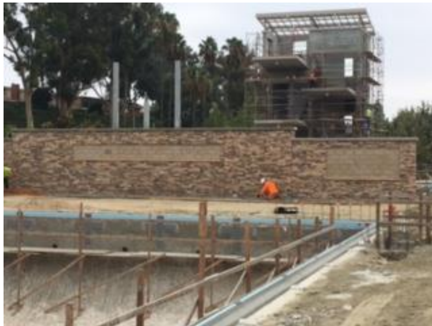
Stone being placed on the wall for Score Boards and Wall of Recognition
