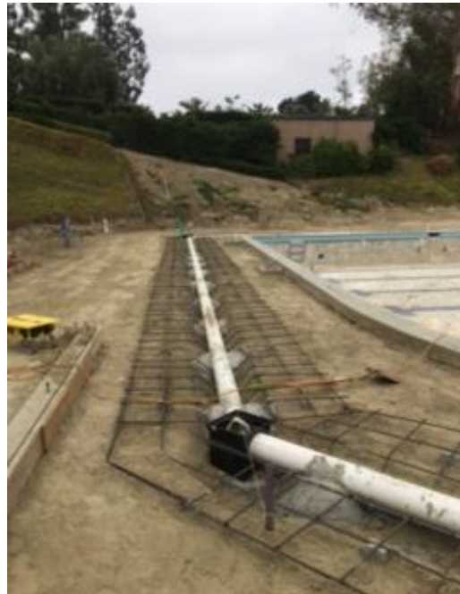
Deck Drains in the Activity Pool Decking
